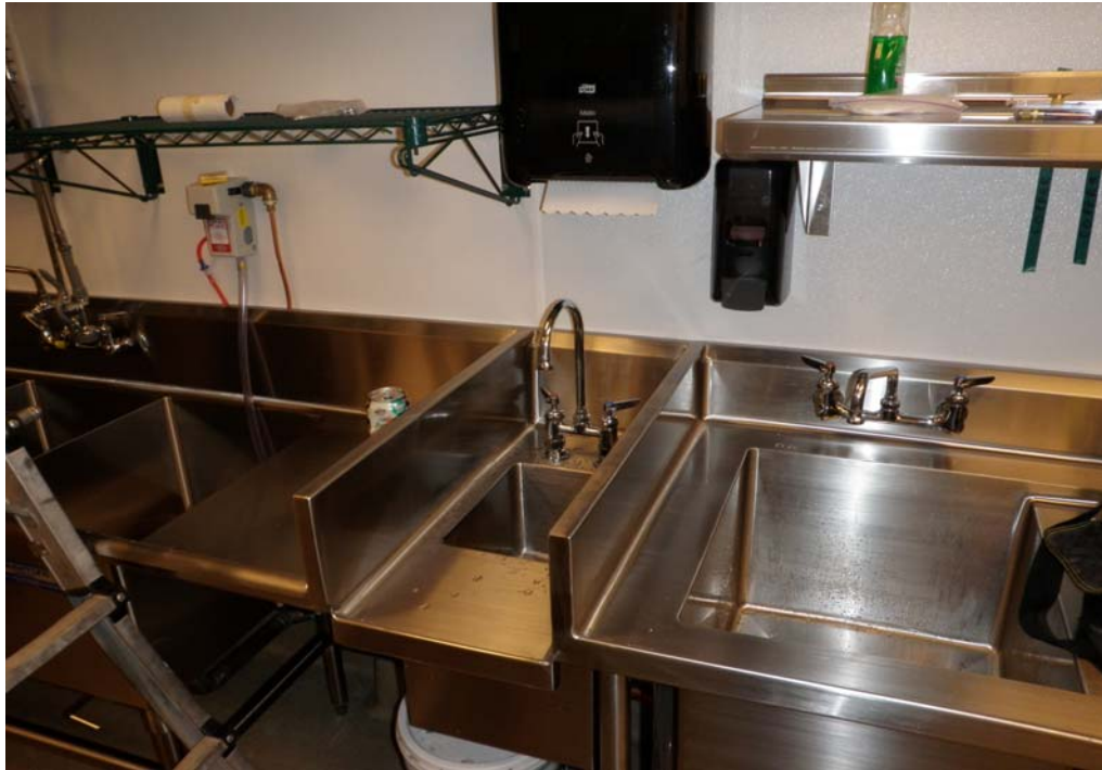
Typical hand-sink installation with splash guards in between
