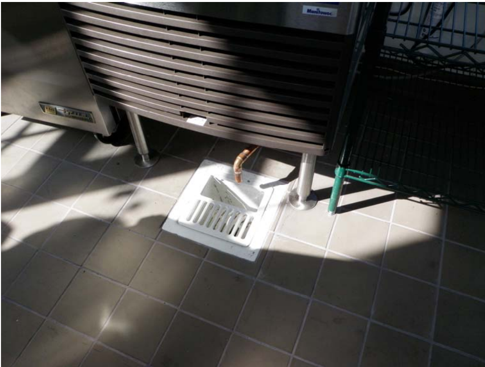
Indirect waste drain connection for an Ice machine (floor-sink flushed to the floor)
